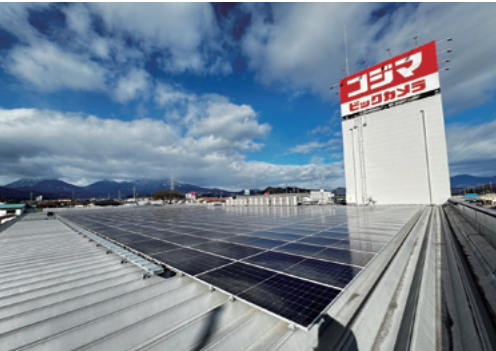
Solar panels installed on store rooftops
